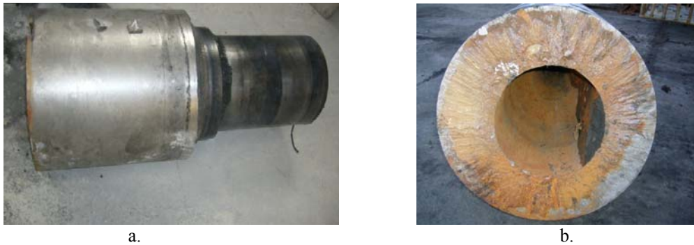
Fig. 4. The refining cylinder and the way it breaks due to cracking corrosion a – presentation of the refining cylinder, b – cracking wear which occurs for the refining cylinders
