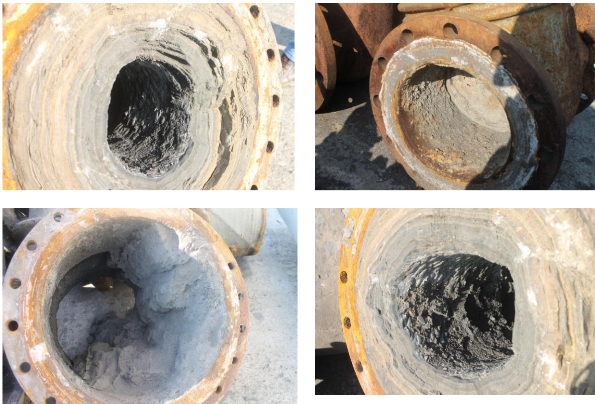
Fig.3 Aspects of corrosion residue deposition
