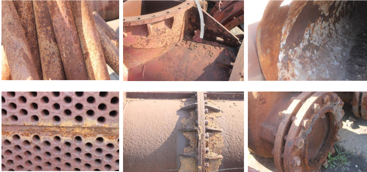
Fig.1. The action of the corrosive environment on steel structures
