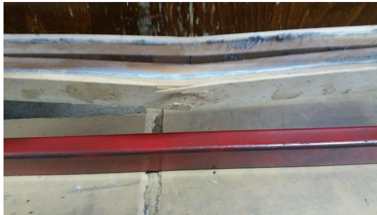
Fig. 4 Tension failure of a reinforced ash wood beam with two GFRP sheets and two slides of beech wood (up and down)
