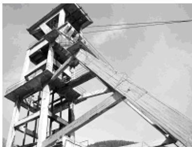
Fig. 1. Installation tower „Auxiliary well no. 2“
