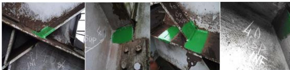
Fig.4. Welds between inclined soles and the top and bottom plates of the platform.
