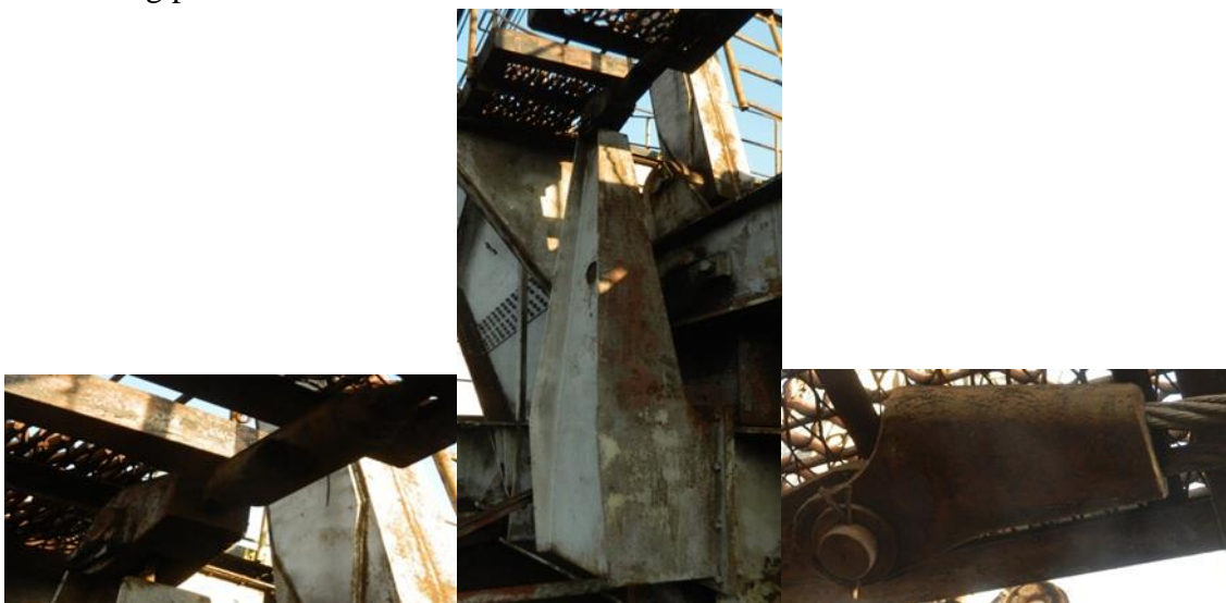
Fig.2 Photos with defects
