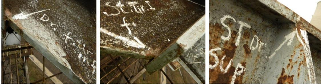
Fig.3 Rust attacked the paint
