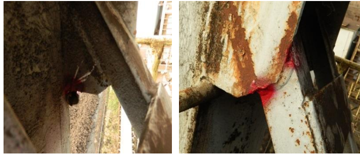
Fig.4 Welding with with marginal burns
