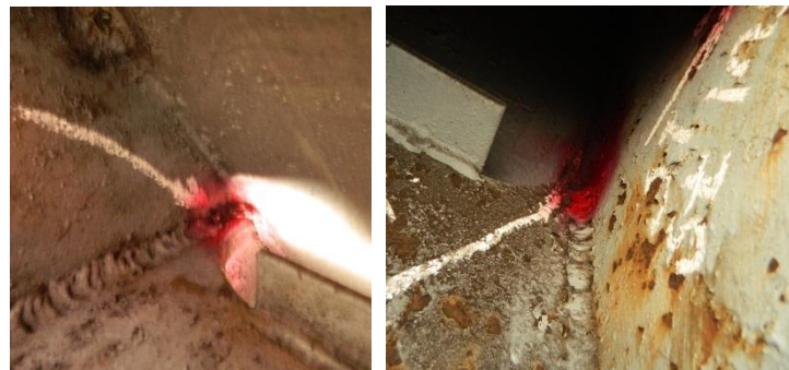
Fig.5 Incomplete welds in hard-to-reach areas
