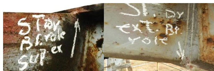
Fig.4 Incomplete welds to support the top and bottom of the roller battery on the mast.
