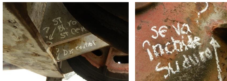
Fig.3 Incomplete welds to support the upper part of the roller battery.
