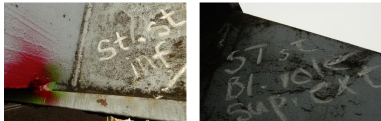
Fig.2 Incomplete welds to support the lower part of the roller battery
