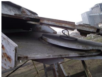
Fig.8 The rust that attacked the paint on the front of the mast beam on the outside.
