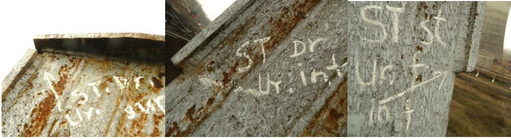
Fig.5 The rust that attacked the paint from the front of the mast beam on the outside
