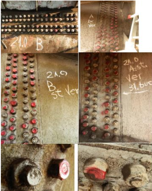
Picture 7. Checking the screws used in the connection between the support skeleton and the tripod supports
