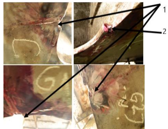
Fig.2. Bottom plate - welding defects.
