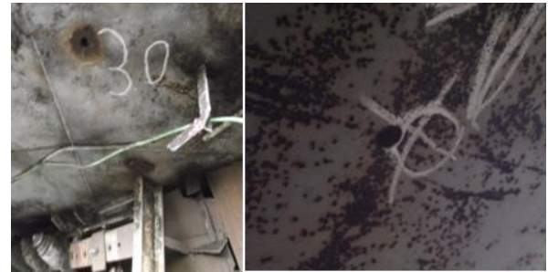
Picture 2. the wrong workmanship of the rainwater drainage holes.
