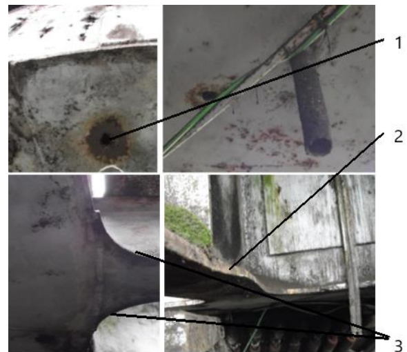
Fig. 1. Leak holes on the bottom plate: 1-drainage holes; 2- limitation bearing ;3-ray connection
