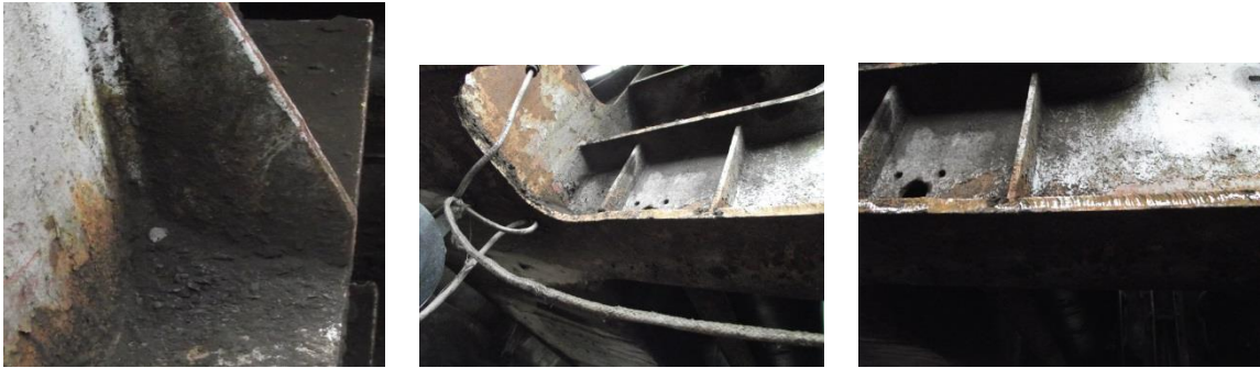
Fig.6 b. Welded joints with rust
