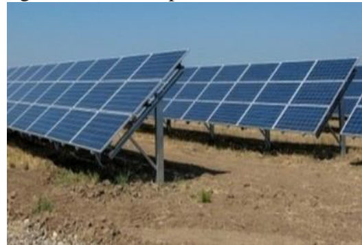
Figure 1 Photovoltaic park with fixed panels
