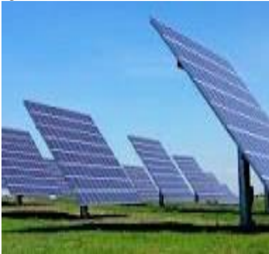
Figure 2. Photovoltaic park in tracking system with one axis
