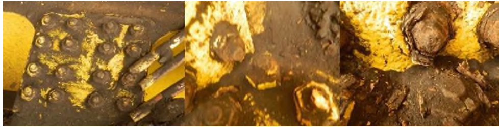
Figure 4. Wear of the screws in the joint area of section II with section III.
