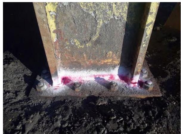
Figure 8- Examination of the welded joint of the base plate - column node 8` and 8
