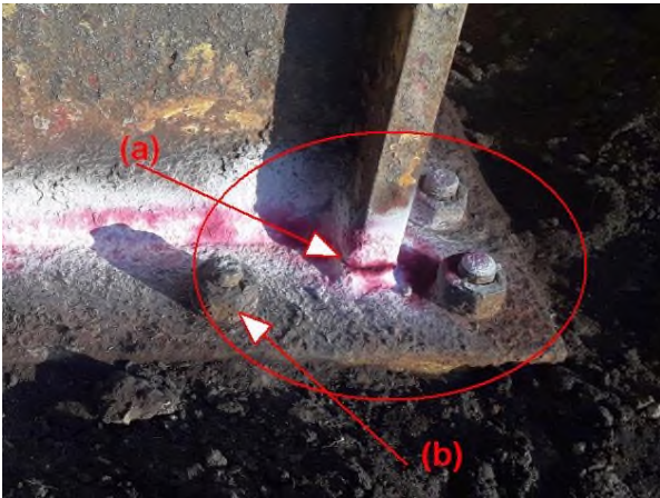
Figure 10 a. Crack on the base plate-pillar; b. Damaged screws
