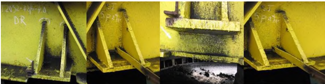
Figure 2. Nonconformities in marked areas.
