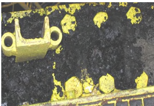
Figure 5. Improper welding of metal structures.
