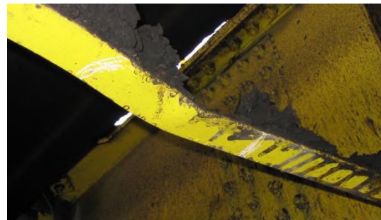
Figure 7. Non-compliance - transverse beam
