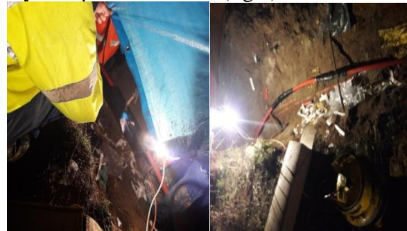
Figure 5. The final stages of repairing the defect: a) The operation of mounting the sleeve in conditions of high humidity ; b) Removal of the tailings from the cable route and laying in the sand of the portion of the cable sleeved
