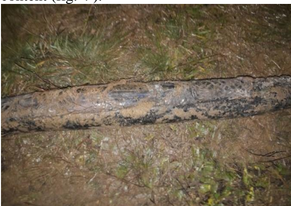
Figure 4. The place of penetration of the shrinkable sleeve as a result of the degradation of the external insulation
