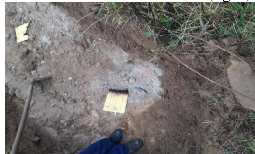
Figure 2 . Identification at the site of the defect of a layer of sterile sand (white) that was also observed along the cable path in the stripped portion
