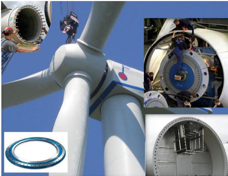
Fig. 7: Bolted Joints at a Wind Turbine
