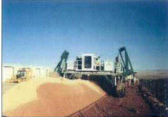
Fig.3. The process of mixing / aeration at a station in bioremediation
