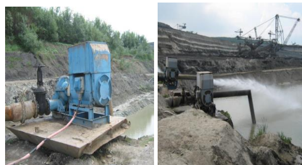
Figure 2. Pump station located in upper layer V and career
